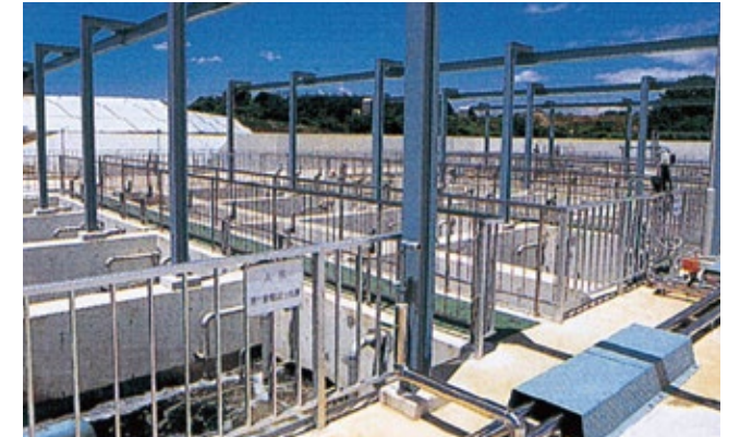
Wastewater treatment facility (contact aeration tank)
