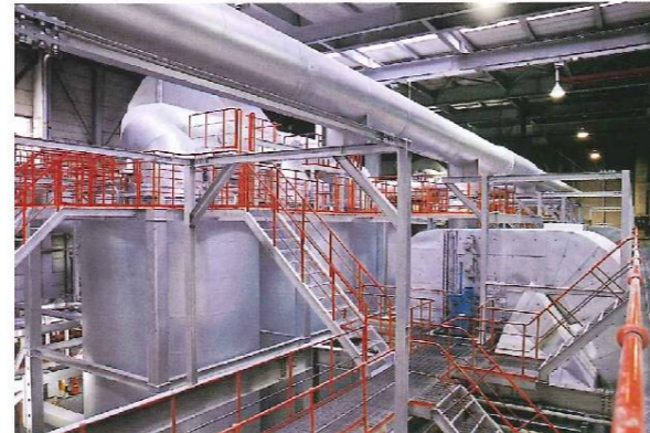
減温塔/Cooling tower
