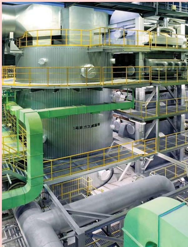
排ガス減温塔・エコノマイザ Exhaust gas cooling tower・economizer
