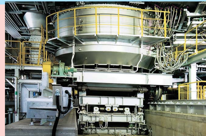
溶融炉本体 Fusion furnace
