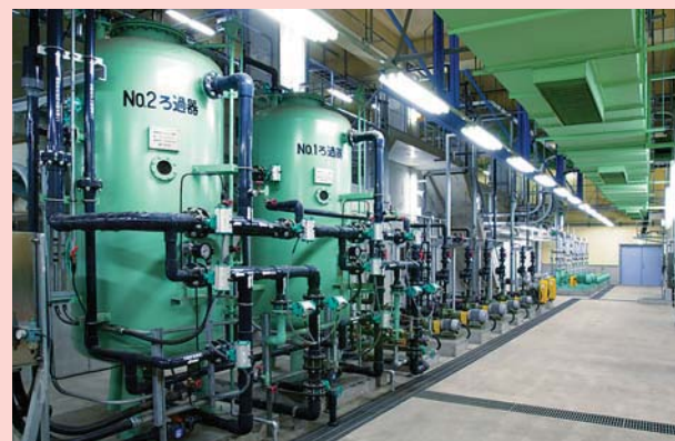
排水処理設備 Waste water treatment system
