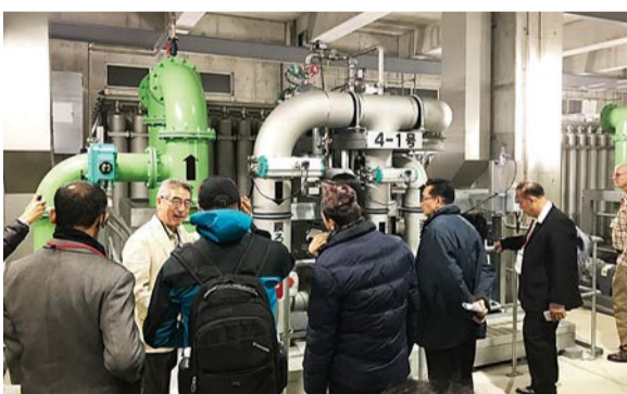
Tour of the Kawai Purification Plant by ADB representatives
