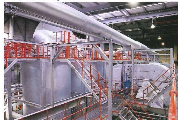
減温塔/Cooling tower
