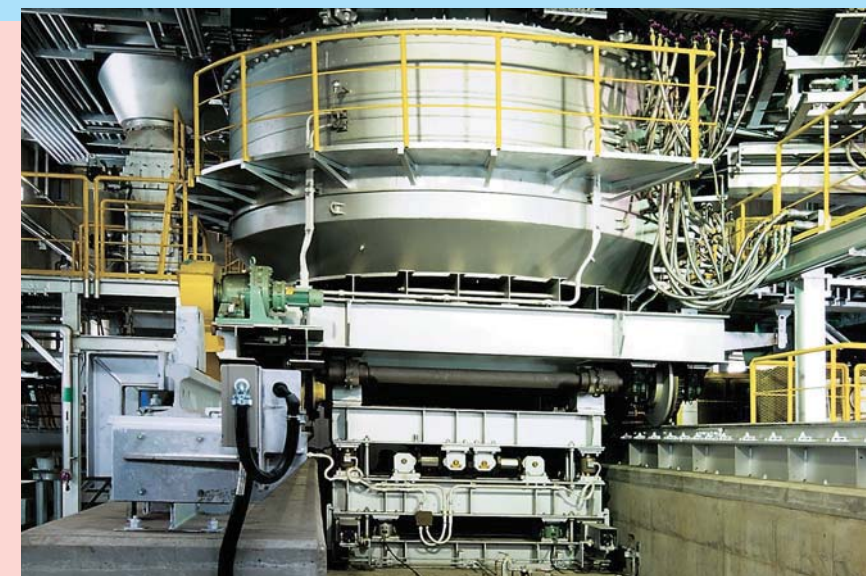
溶融炉本体 Fusion furnace
