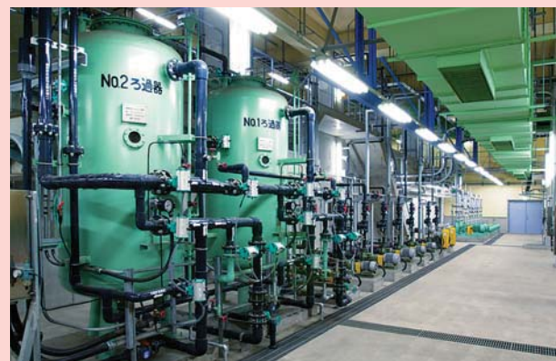
排水処理設備 Waste water treatment system
