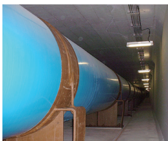
1,350 mm-diameter water pipe inside the utility tunnel
