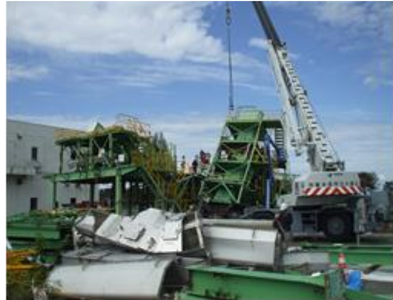
Damaged grit separator
