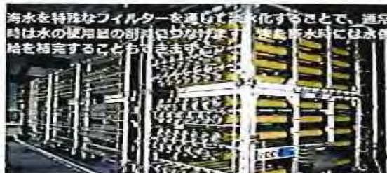
Kitatani purification plant - Okinawa
